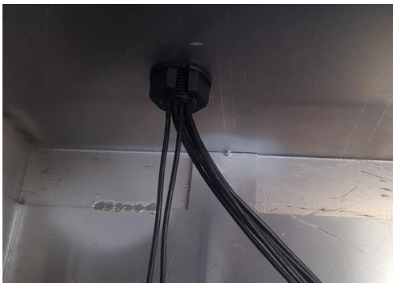
Figure 20: View of the antenna from inside the cabinet
