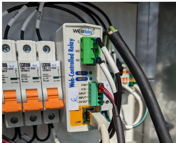
Figure 25: Power and ethernet on the Power DIN Rail
