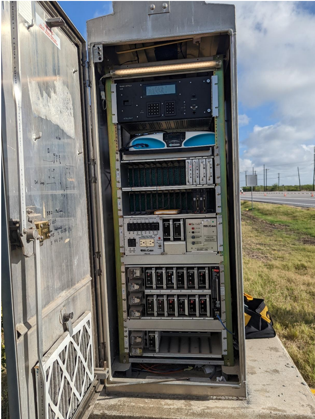
Figure 37: Front view of 332 cabinet after installation.
