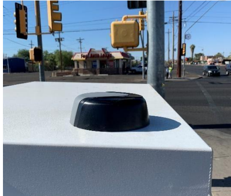
Figure 19: Antenna mounted to top of cabinet
