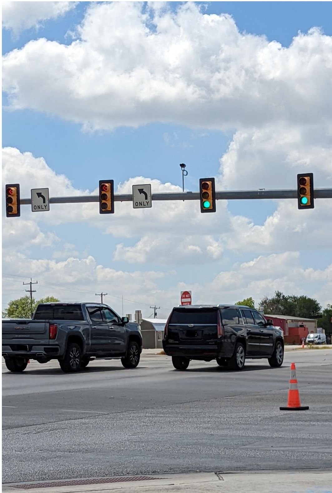
Figure 41: Sensor unit installed at one approach
