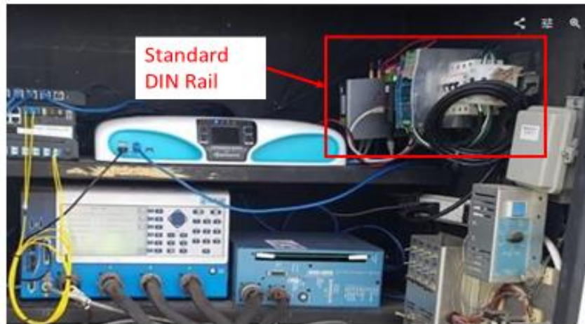
Figure 17: Installing the CU and Standard DIN Rail
