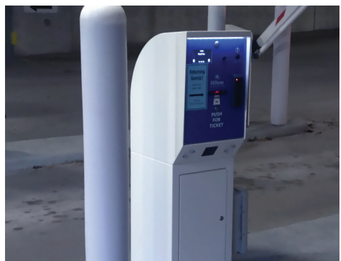
After TIBA Parking Systems installation, the parking garage at the Milwaukee Hilton provide exceptional 24/7 guest experience without breaking down.
