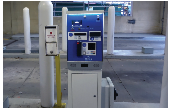
TAPCO installed this TIBA Parking Systems Point-of-Sale terminal inside the Milwaukee Hilton location.
